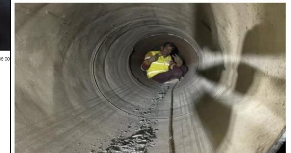
When excavators and powerful drills had failed to bore through the debris, the work was eventually assigned to 12 "rat-hole miners," who was tasked with digging away at 12 metres of rubble. Image Courtesy: @jayanta_malla/X
